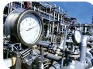
Condensate line pressure gauge BEFORE GEM Traps (175 PSIG)
